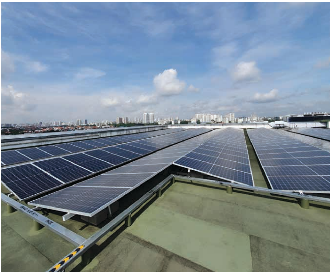
Figure 11: Sinenergy – EPC Project
